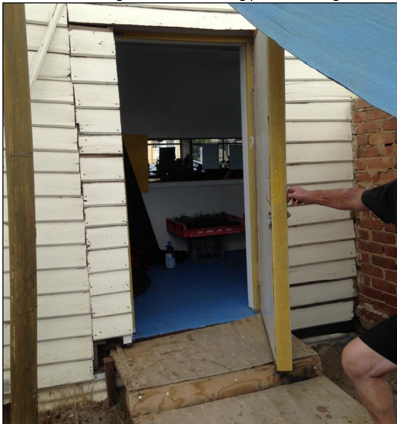
Access door for carers at back of building looking through to public viewing window
